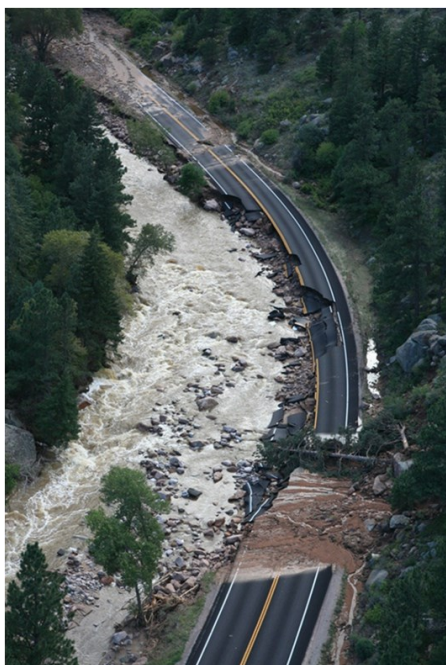
Flooding caused severe damage to state and local roads. Although some of the most extensive damage occurred to roadways through mountain canyons (left), as flood waters moved east, roads and bridges in the plains were impacted as well. SH 66 is shown below.
